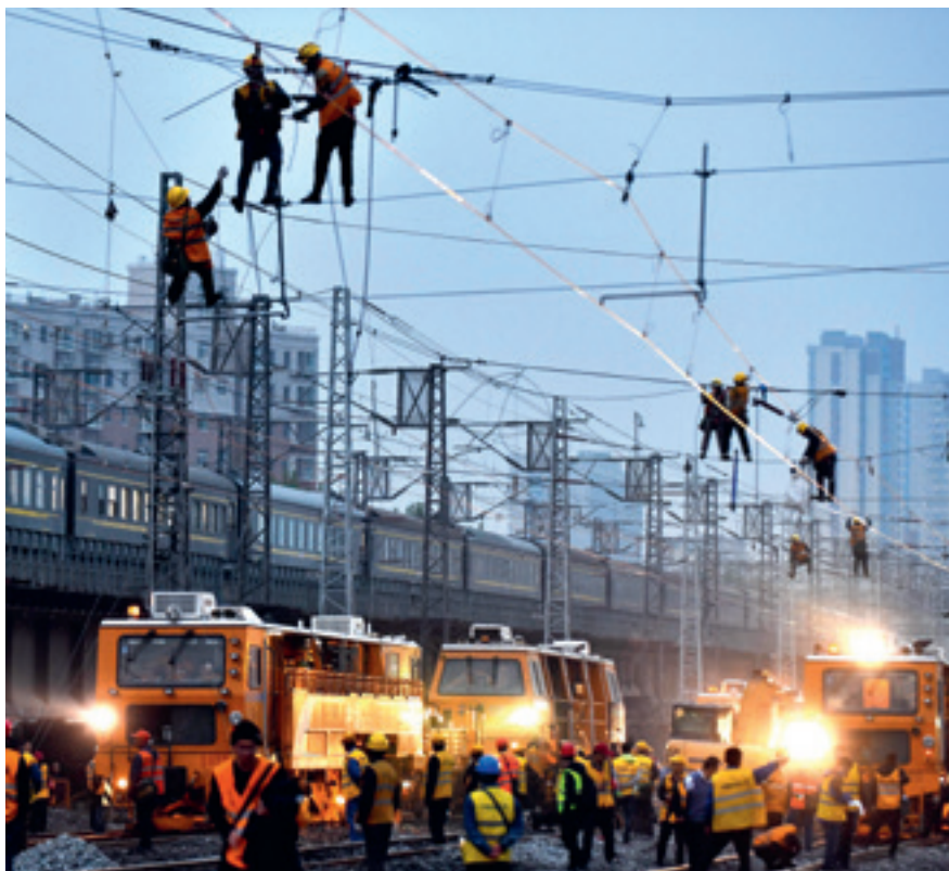
The site of a railway reconstruction project in Jinan, Shandong Province, on April 12
